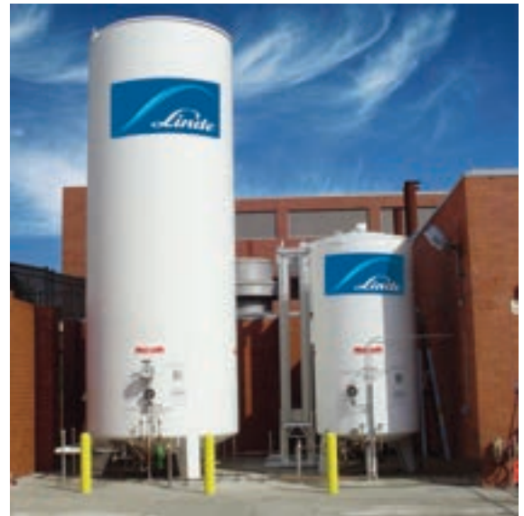
Figure 4: Medical Bulk Gas Installation
